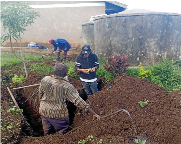
RWHT connection to active Gravity Flow Scheme at Karungaya Primary School.
