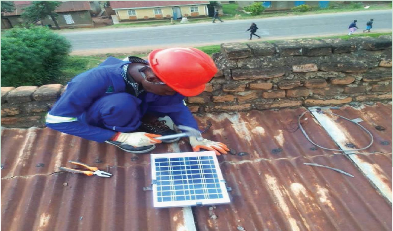
Joash Masereka a Solar installation, repair, and maintenance trainee installing a solar panel in Kasese.
